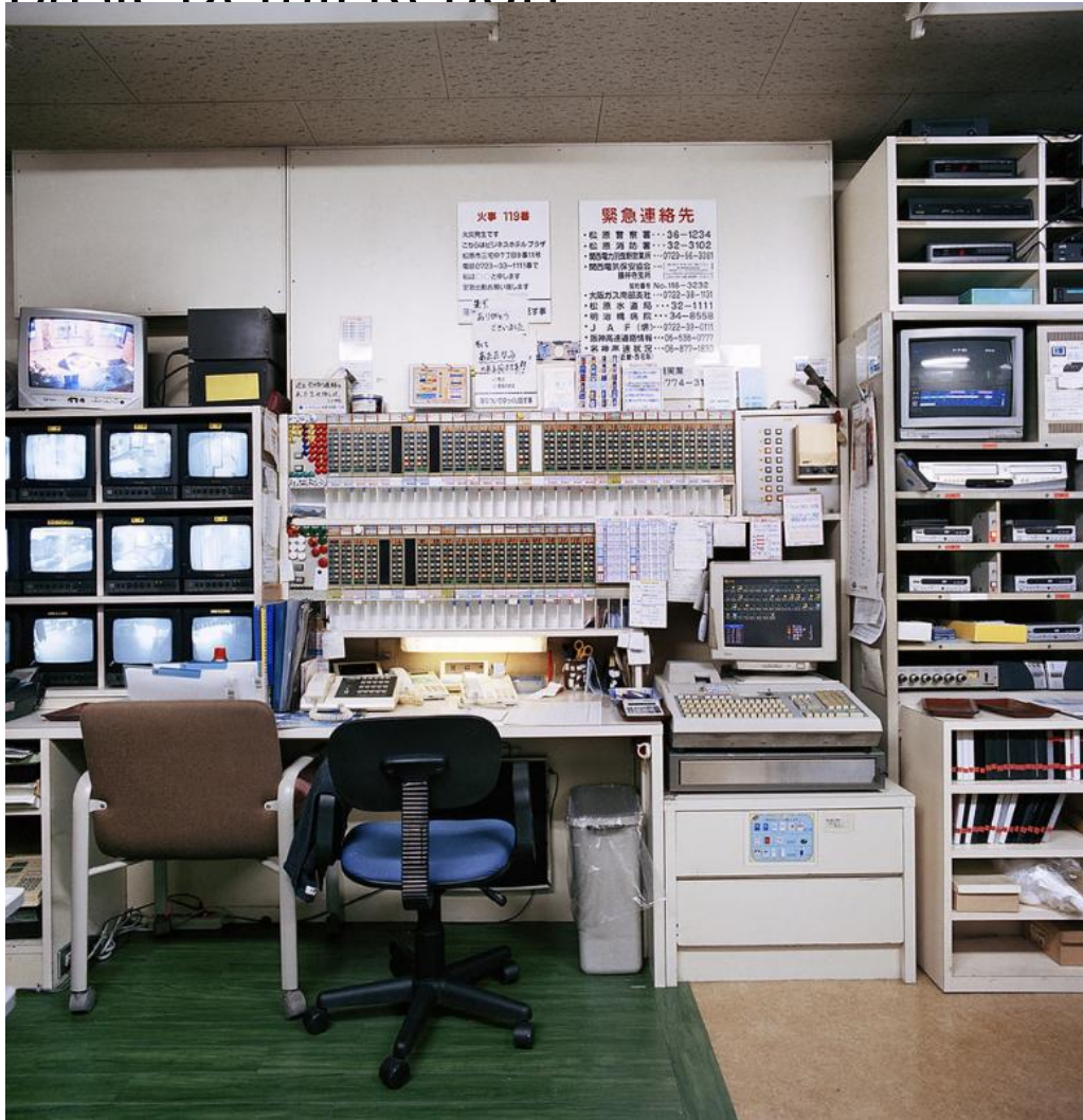
Title Control Room, Hotel Plaza, Osaka
